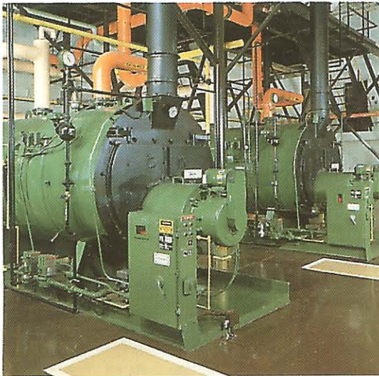
Central High School – Saginaw, MI (2) 150 HP Natural Gas Burners, Hot Water Generators
