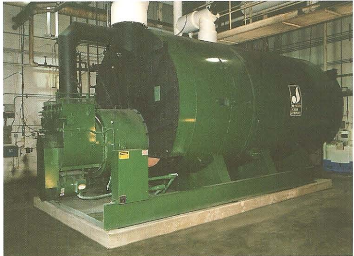
Acco Chain and Lifting Products – York, PA (2) 750 HP Natural Gas/Propane Burners, High Pressure Steam
