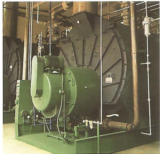
Pilgrim's Pride – Mt. Pleasant, TX (1) 2000 HP, (1) 1200 HP, (3) 800 HP Natural Gas/Fume Burners, High Pressure Steam
